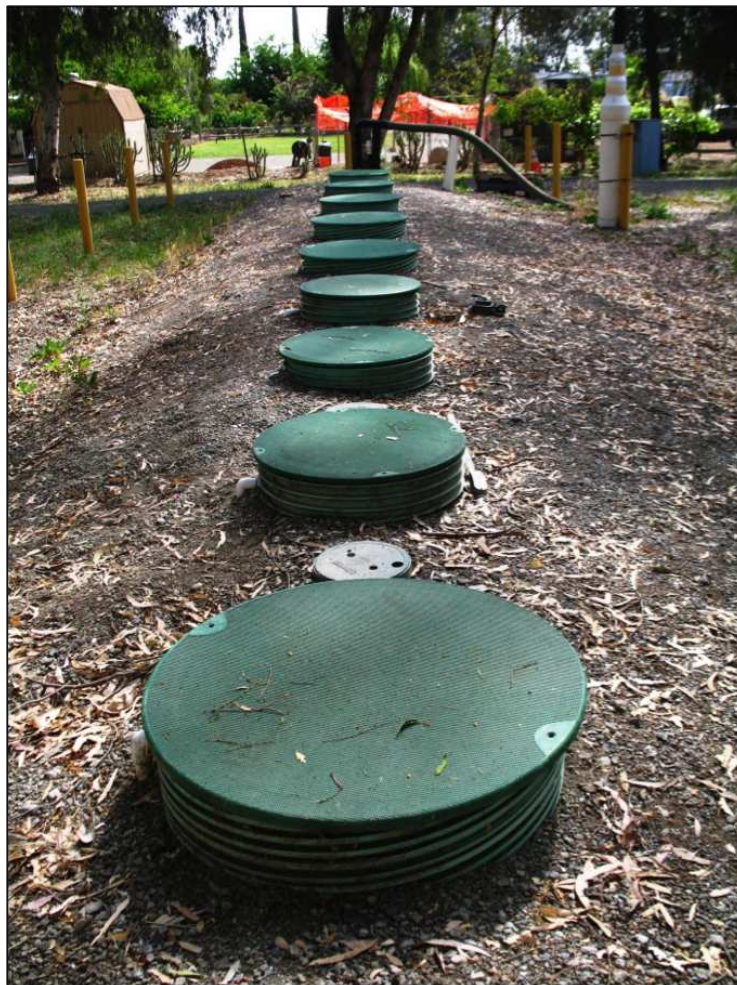
Figure 4. A nine compartment anaerobic baffled reactor (ABR) in operation, Dunnigan, California, USA (photo reproduced with permission of Stewart Oakley).
