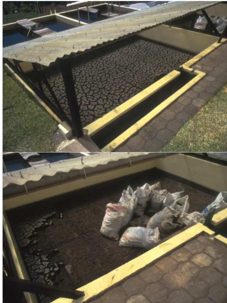
Figure 5. Sludge drying beds for the wasted upflow anaerobic sludge blanket (UASB) sludge at Sololá, Guatemala. The sludge is well digested and dried and is currently provided to the public in bags as a soil conditioner and fertilizer. This practice should be prohibited until there is sufficient removal of pathogens in the sludge. Dewatered sludge should be treated for pathogen removal prior to reuse (see Sludge Management Chapter) (photos reproduced with permission of Stewart Oakley).
