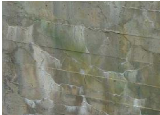
Figure 2. 2: Extensive cracking and stains at the Tascaván dam gate (ARAÚJO, 2008 apud GOMIDES 2009).
