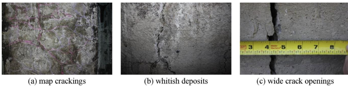
Figure 2. 10: Symptoms of deteriorated concrete foundation. (ZHONG and WILLE, 2018)
