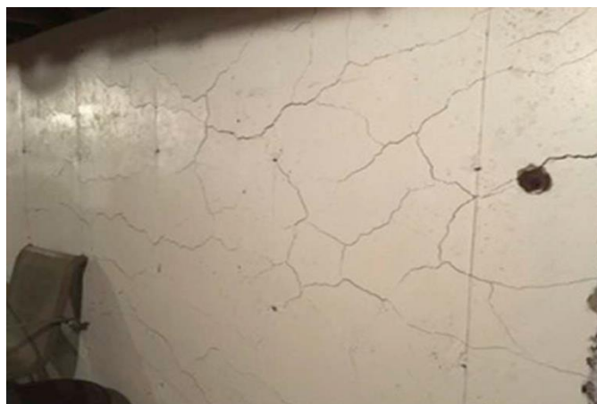
Figure 2. 9: Basement wall affected by internal sulfate attack. (GEISS and GOURLEY, 2019)
