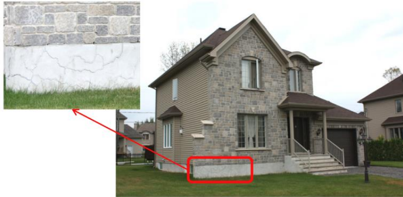
Figure 2. 6: Extensive cracking on the foundation blocks of a house in Quebec, Canada (RODRIGUES et al. 2012b).
