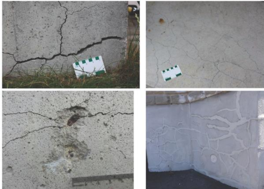
Figure 2. 7: Typical degradation signs observed in foundation concrete containing sulfide-bearing aggregates in the Trois-Rivières area (RODRIGUES et al. , 2016b)
