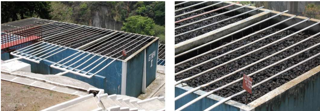
Figure 5. A volcanic rock trickling filter with a fixed hydraulic distribution system. This system has been in operation for 35 years with an average daily flow rate of 500 m 3 /day. Filter located at the University of San Carlos, Guatemala City, Guatemala (photo by Stewart Oakley)
