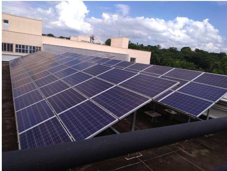
Figure 2-12 - Photovoltaic panels installed in the photovoltaic solar power plant Tesla
