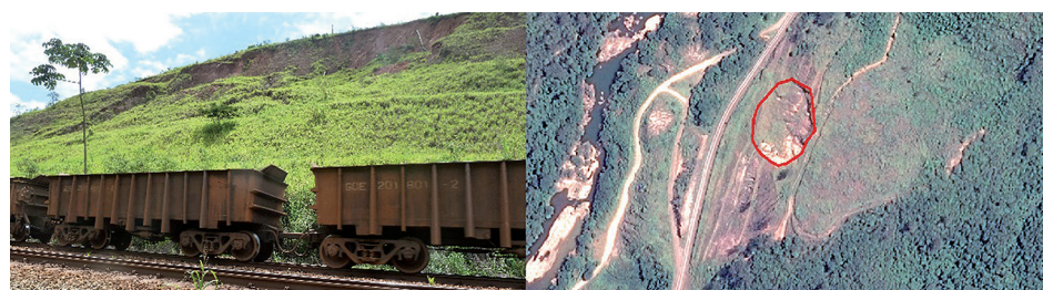
Figure 1 Partial view of landslide's scar in stretch 493+600 of EFVM (left). Image of the year 2016 from Google Earth Pro of stretch 493 + 600 with polygon marking the scar (right).
