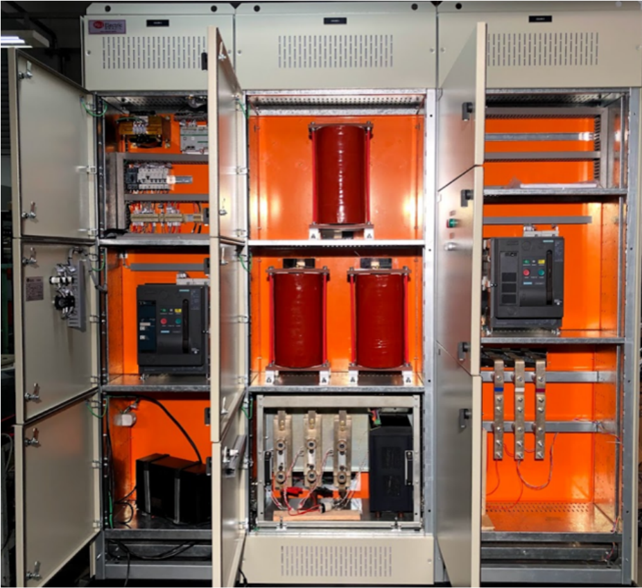
Figure 4.70 Real switchgear prototype.
