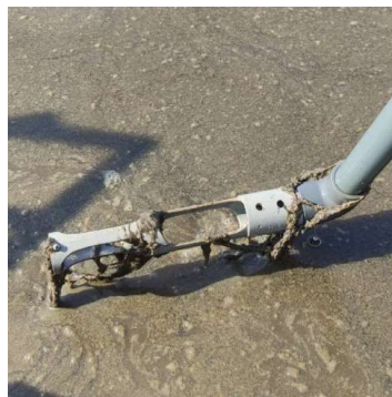
Figure 60 – Solids accumulation on the ultrasonic sensor after one week (RWZI Grou)
