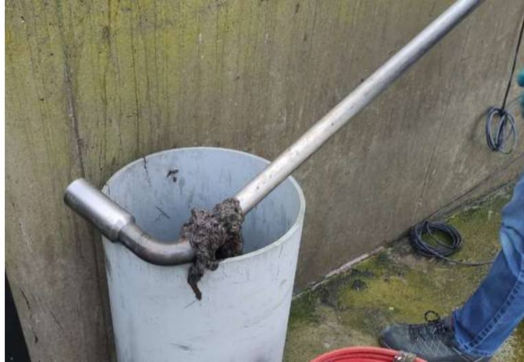
Figure 59 – Solids accumulation on the optic sensor (RWZI Grou)
