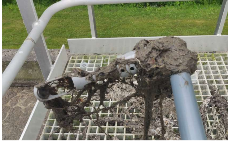
Figure 64 – Solids accumulation on the US sensor after two days - RWZI Leeuwarden
