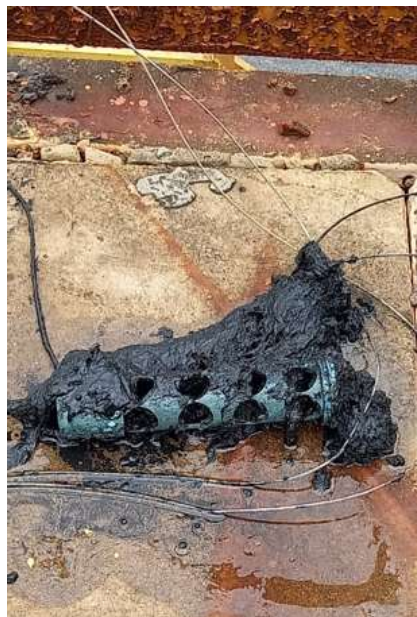
Figure 45 – Solids accumulation on the US sensor after two months inside the UASB reactor from ETE Betim Central
