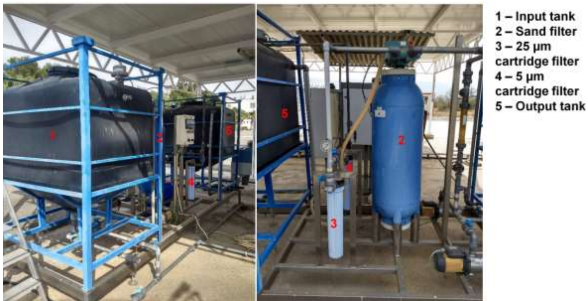
FIGURE II.3.11 – Effluent filtering unit: sand filter and cartridges microfilters (25 and 5 µm)
