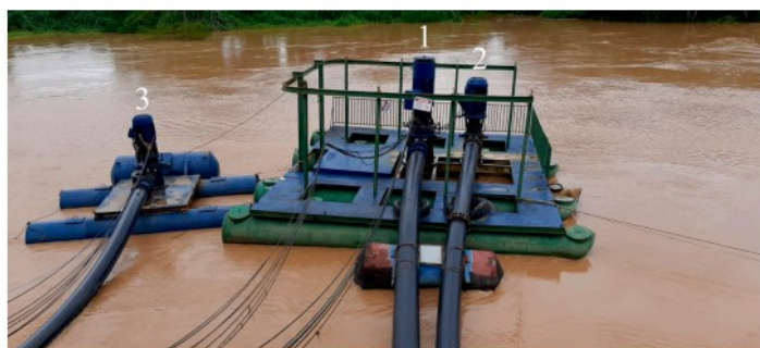
Figure 2. Elevated Pumping Station II, Rio Branco, Acre, consisting of a set of vertical turbine-type pumps. Note: 1—Pump 1; 2—Pump 2; and 3—Pump 3.
