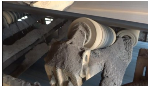
Figure 1. Dirt buildup on belt conveyor roller structure.
