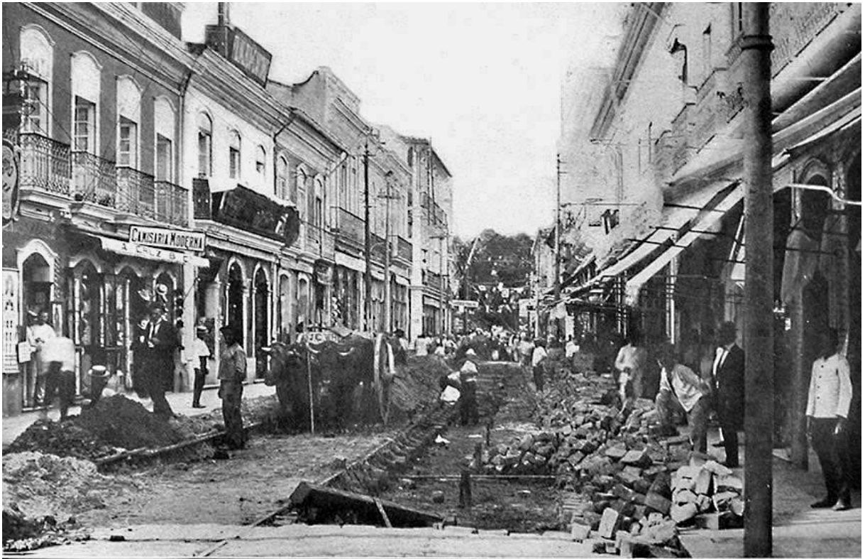
Para Tramways—Old Track and Excavation for New Track on Rua C. Joao Alfredo
