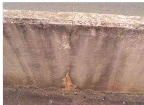
(f) Manchas e fissura vertical na barreira New Jersey.
