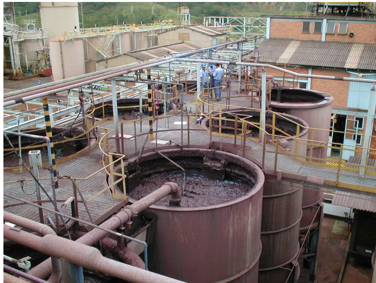
Figure 4.10 - Leaching Pachuca Tanks
