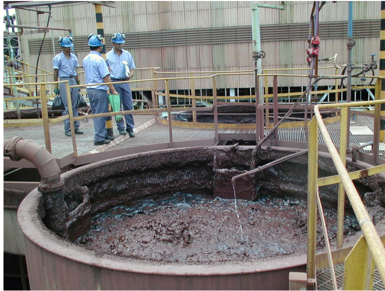
Figure 4.11 - First Leaching Pachuca Tank where Cyanide is Added
