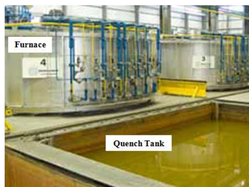
Figure 3.69 – Tanks for quenching of hot rolled rings (Rotek® Rings, 2011).
