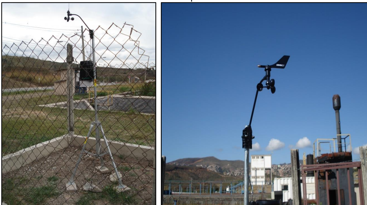
Figure 5.10 - Meteorological Station installed at CePTS for onsite monitoring of various environmental parameters.
