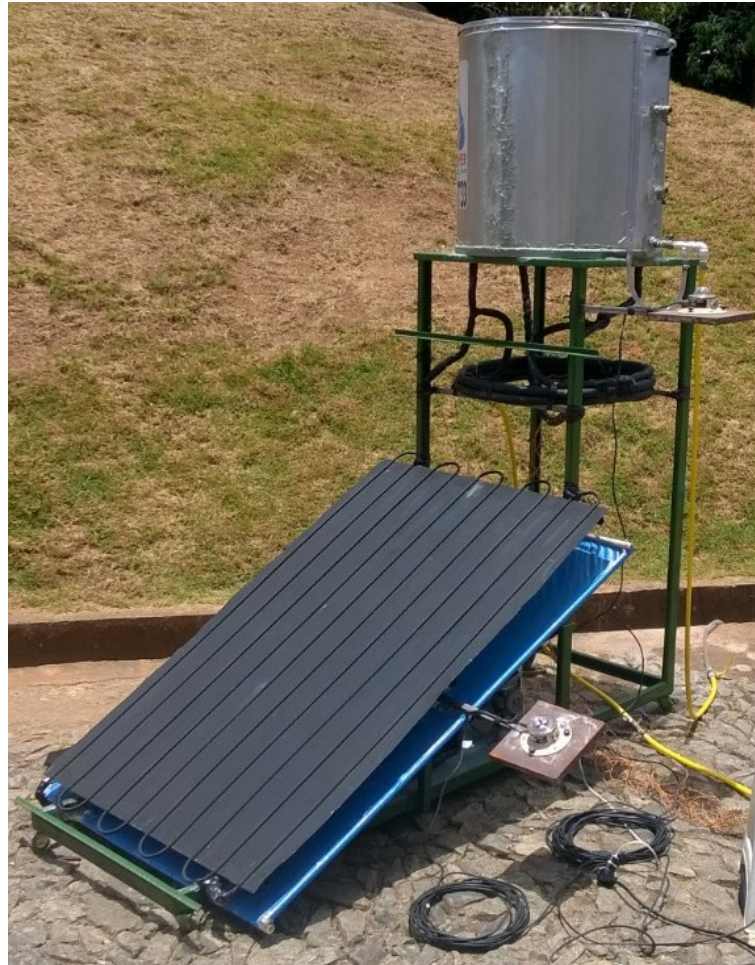
FIGURE 4.1: Photo of the R134a DX-SAHP installed at GREA of UFMG.
