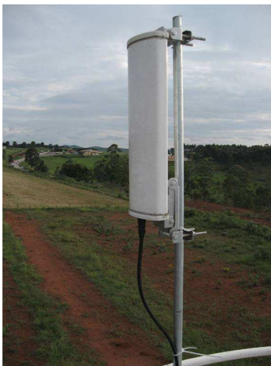
Figura 3.18. Antena painel setorial instalada
